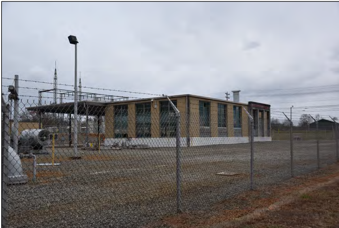
Figure 2.3.7. Plantation Pipe Line Pumping Station, facing northwest.
