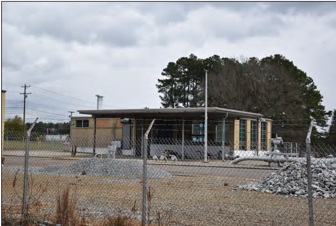
Figure 2.3.5. Plantation Pipe Line Pumping Station, facing south.
