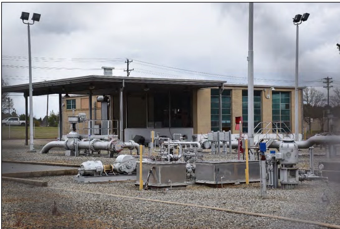
Figure 2.3.6. Plantation Pipe Line Pumping Station, facing southeast.
